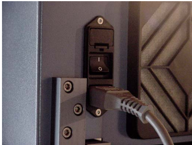
Photo 1-0 General power switch
